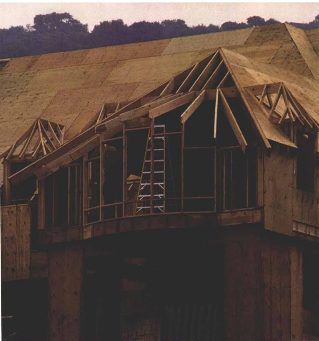
With half the common rafters in place, the curve of the eyebrow roof begins to take shape.
