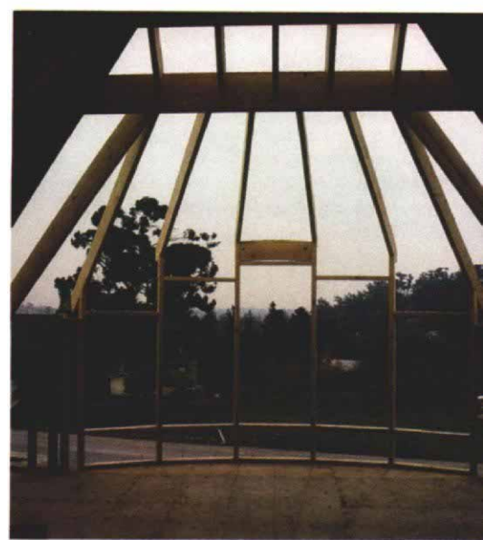
A 4x12 header secured to the roofs hip rafters carries the upper ends of the common rafters in the eyebrow roof. At the wall, every other rafter bears on a king stud. The chalklines on the floor were used to calculate the run of each rafter. In the center bay of the window, one segment of the arched header has been installed just above a temporary spacer.
