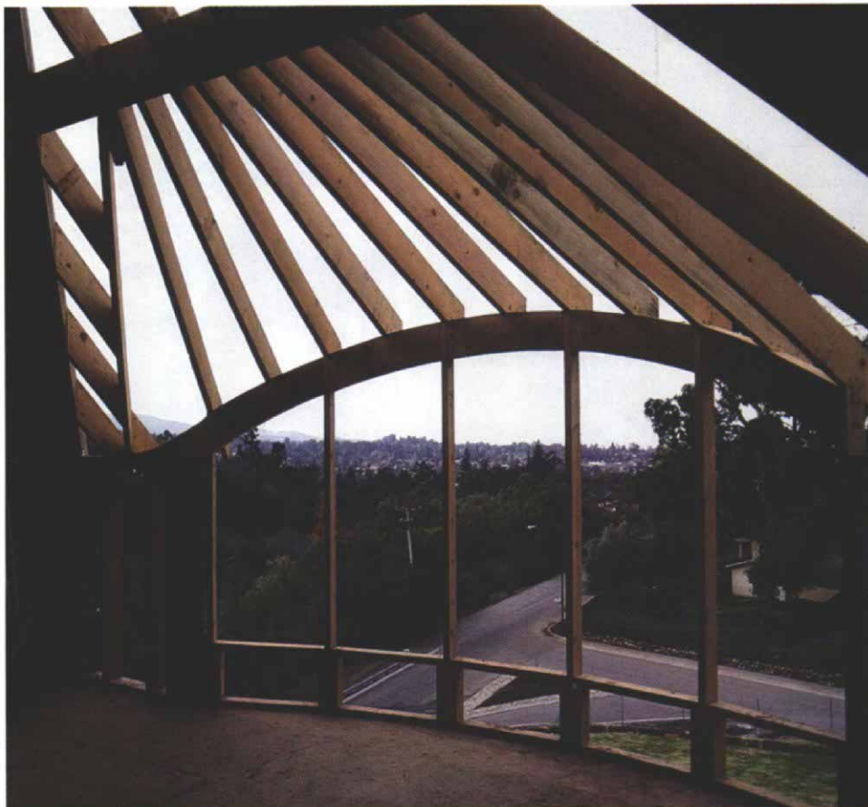
The temporary spacers between the king studs have been removed, and in their place the curved headers define the radius of the eyebrow roof. At the far side, a curved block atop the straight wall makes the transition to the arched form of the bowed wall.
